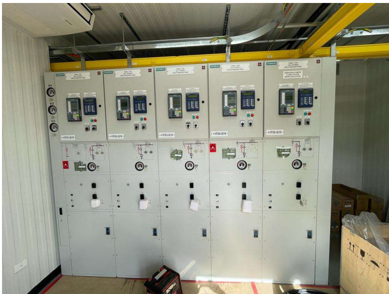
Circuit breakers in the switch room
