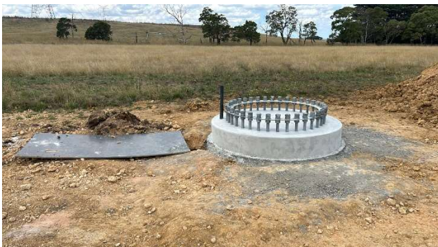
Transmission pole foundation
