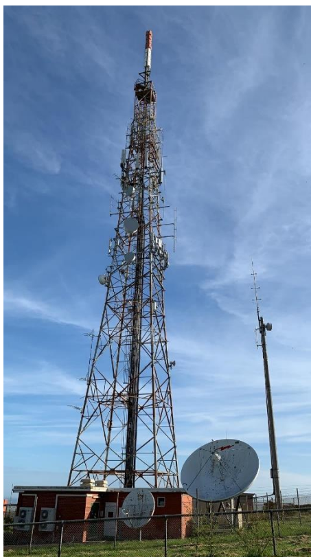
Figure 3-1 Tower Hill – Transmission Tower
